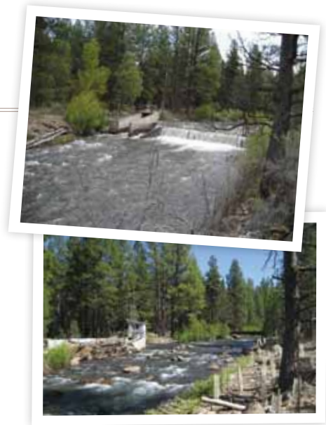
TOP: Before restoration, the Three Sisters Irrigation Diversion dam blocked upstream passage for fish. BOTTOM: With the stream channel built up to meet the height of the dam, fish are able to use habitat upstream.
